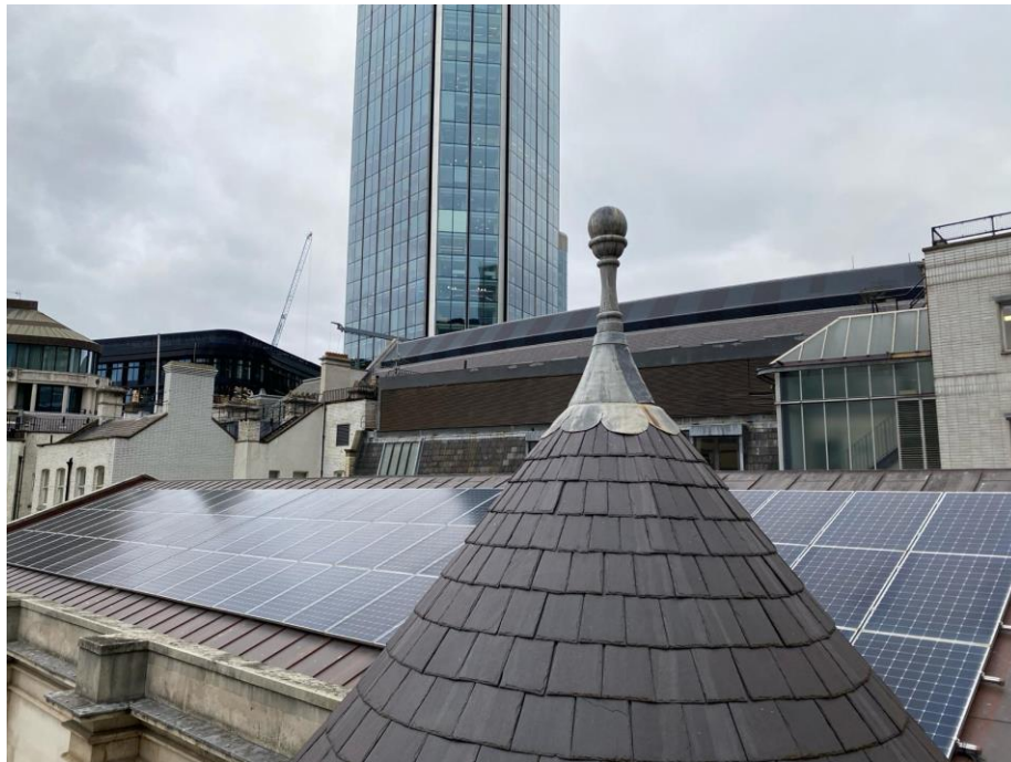
Rooftop Solar Panels At Merchant Taylors' Hall
